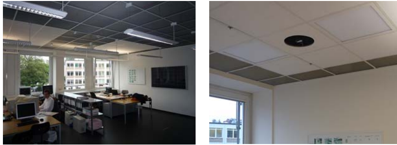
Fig. 3 Pictures of the room (left) and the fan integration in a typical acoustic panel of the suspended ceiling section (right). The major part of the ceiling is now equipped with porous metal meshes as shown on the left picture. A section with acoustic panels remains above the work places to hold the fan combined with two flat LED light panels.
